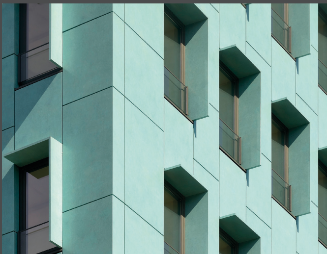
Metropolis, Belgium | Material: ALUCOBOND® PLUS vintage Patina Copper | Architect: A.D.E. architectes | Fabricator: Francovera © Willemen Real Estate
